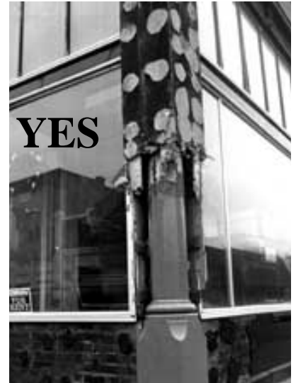
Removing a metal grid installed over an original facade. (Photo: Bob Dunn, NPS)
