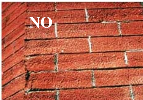
Abrasive cleaning methods, in this case sandblasting, can permanently damage building surfaces. (Photo: NPS files)
