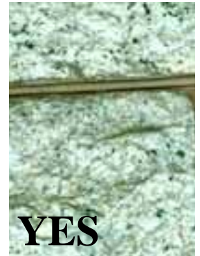
Late 19th century granite that has been repointed with the original joint profile and mortar color. (Photo: NPS files)
